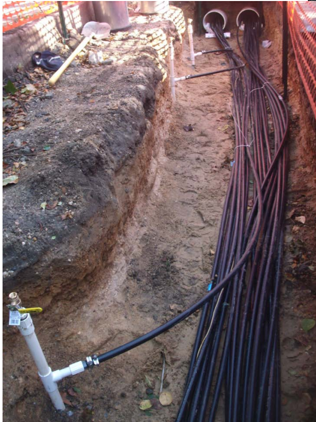
HDPE injection lines feed through conduit that runs under N. Clinton Ave. to the oxygen injection system shed located at 33 N. Clinton Ave.
