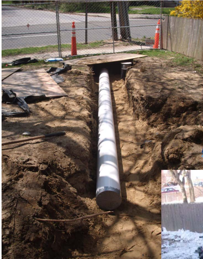
Conduit for HDPE injection lines for Cooper Lane
