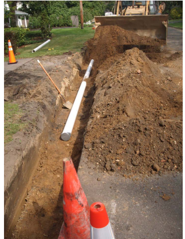
Placing conduit in portion of trench at the end of a private driveway
