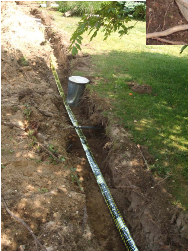
Demarcation tape labeled "Caution Buried Gas Line Below"
