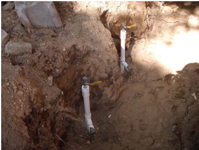
Injection points with fitting connections
