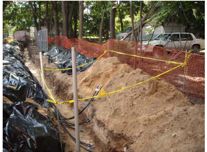
HDPE injection lines leading to shed location
