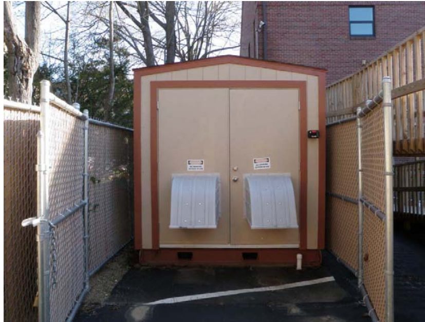
Oxygen Injection System Shed
