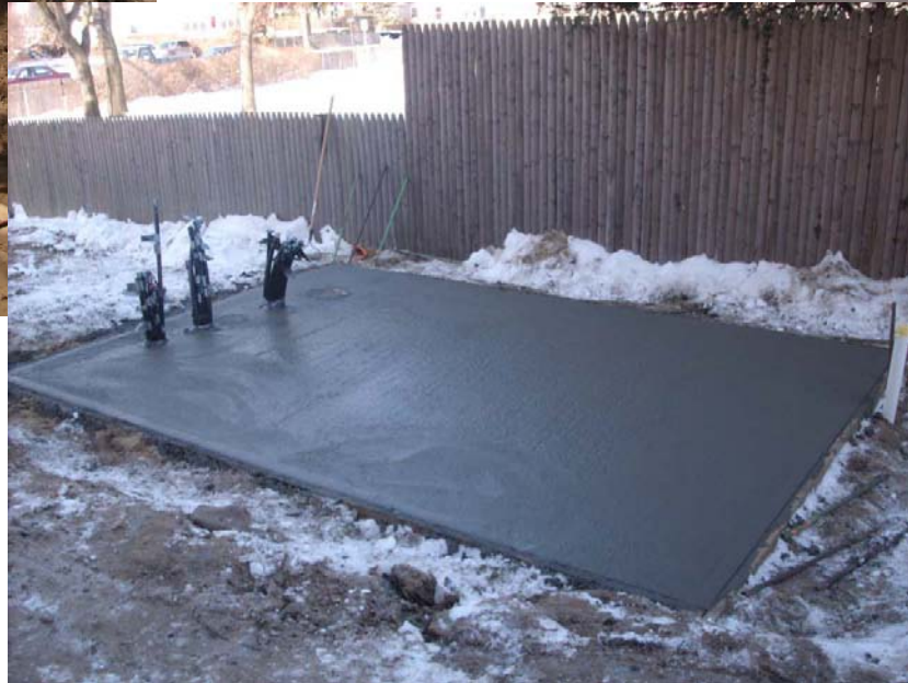
Concrete slab for the injection system shed 33 North Clinton Ave. Photo Log Appendix A
