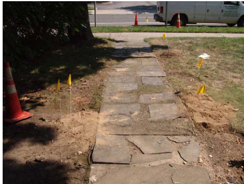
Walkway to N. Clinton Ave. before restoration 34 North Clinton Ave. Photo Log Appendix
