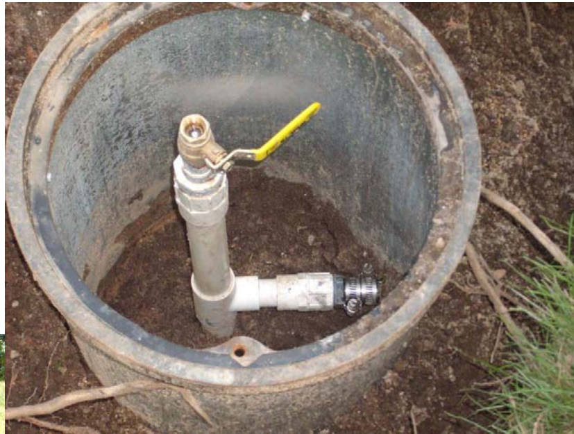
Injection well with connector fitting in curb box
