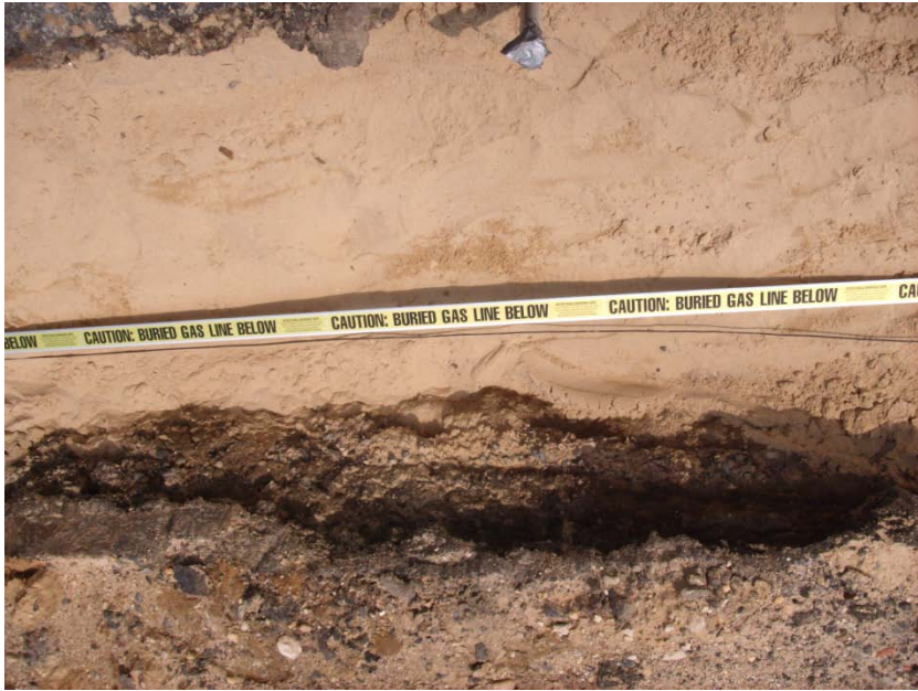
Demarcation tape labeled "Caution Buried Gas Line Below"
