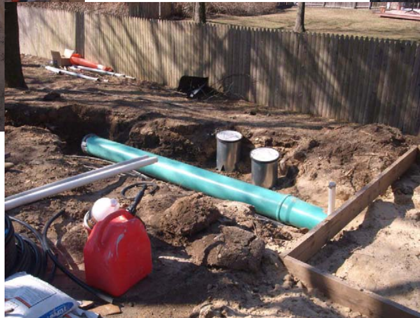
Conduit for Cooper Lane Extension injection lines
